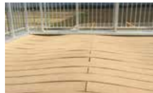
Case example of decking expansion due to water absorption
